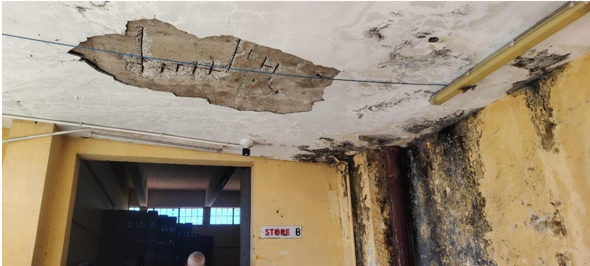
Photo showing structural damage and mold infestation in Store B used for the storage of medicines and medical supplies are kept.
