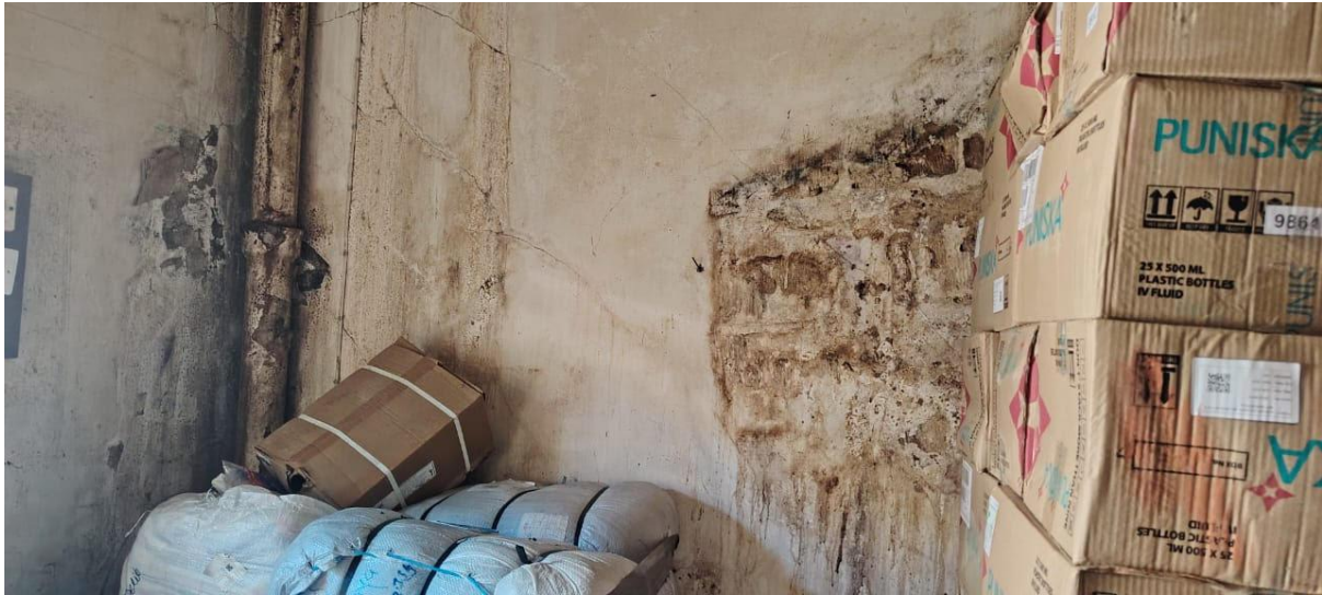
Photo showing mold infestation and humidity damage to boxes.
