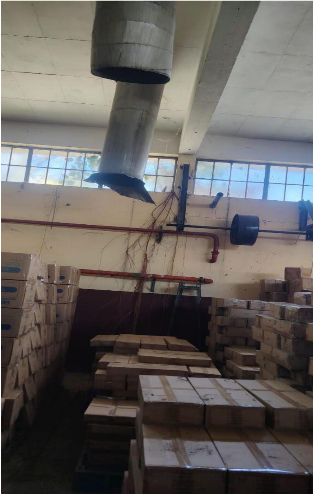
Photo of one of the two former Tobacco Board warehouse showing invasion of banyan tree roots.
